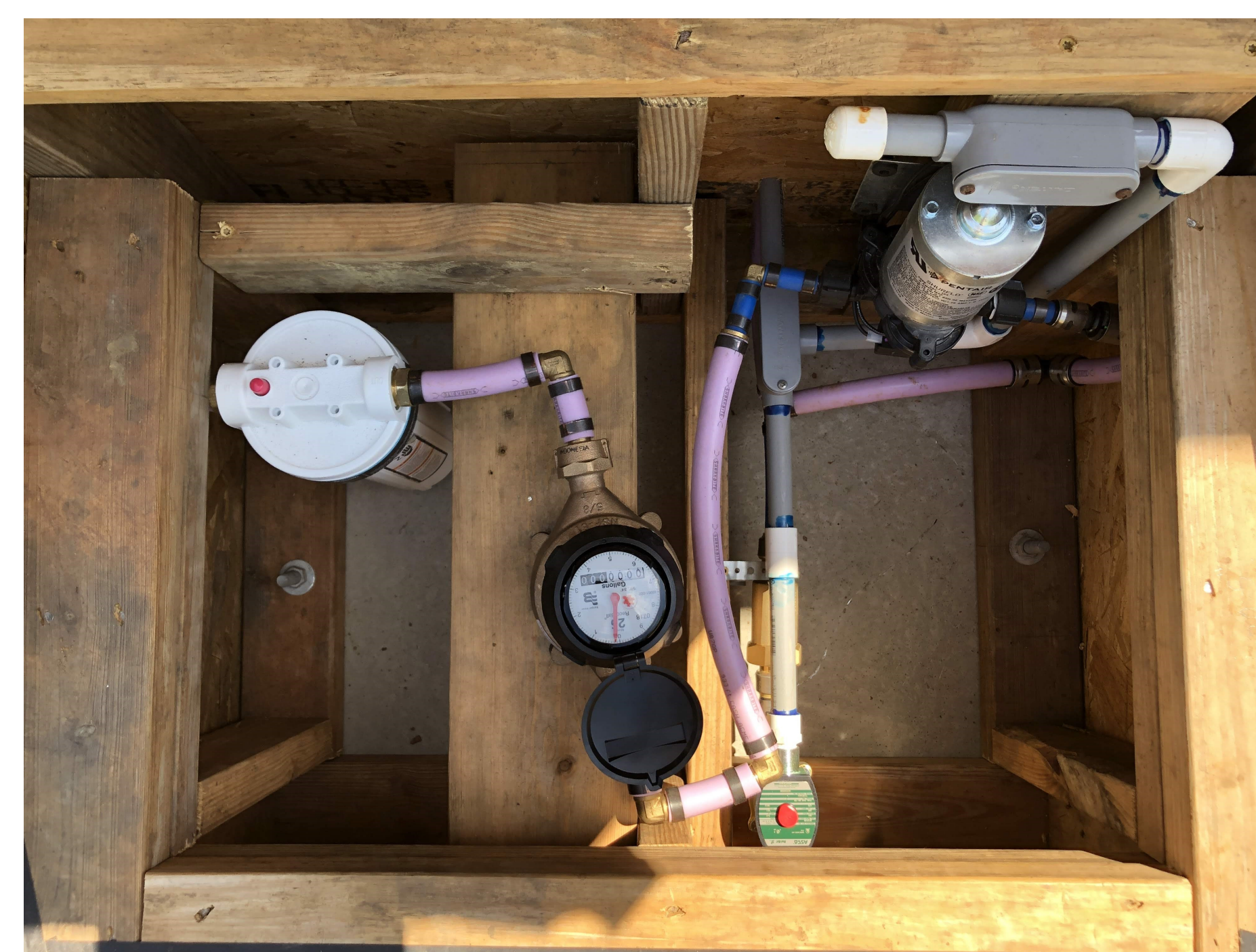
Figure 3 - Completed pump and filter system.
