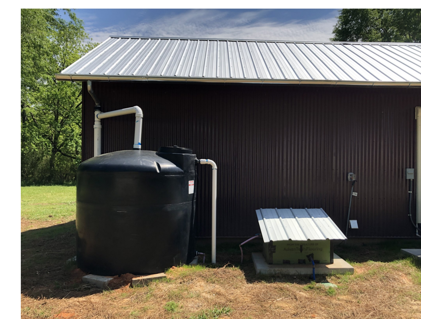
Figure 4 - Installed rain catchment tank.
