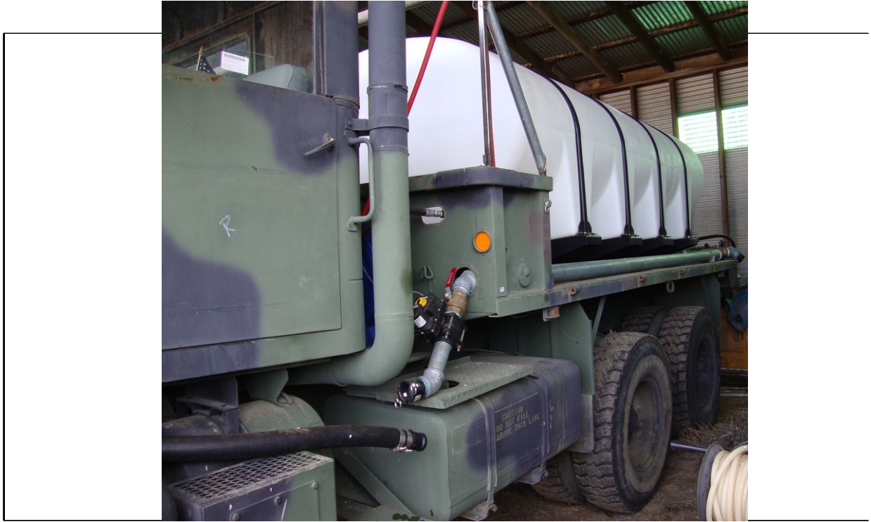
Here is the plumbing going to the monitor on the front of the truck from the pump.
